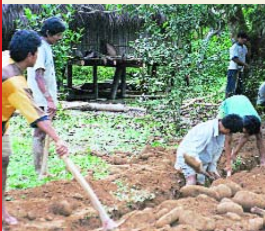
Mayapo community residents dig ditches to lay pipes for their water system.
